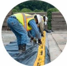
Containment and spill prevention
