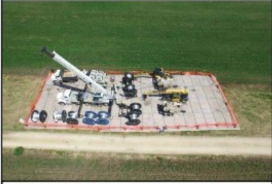
EPZ Grounding System
